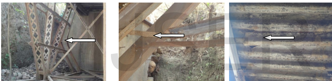
Figure 4 (a)End Member Buckled (b) Inadequate Horizontal stiffener (c) Corroded and damaged Deck
