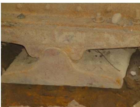
Bearings before Retrofitting
