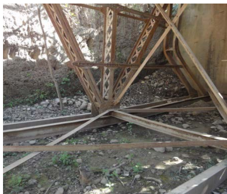
Bottom members before Retrofitting
