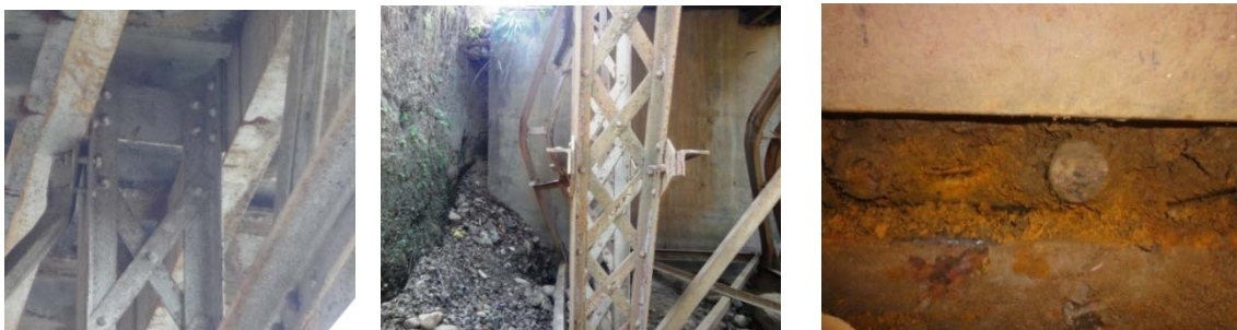
Figure3(a),(b),(c): Loose Rivets, Bearing Filled up with Soil, Roller filled with soil
